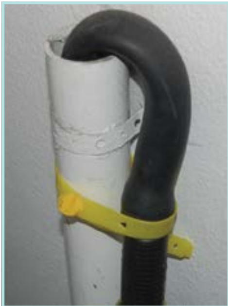
Figure 15. Washing machine drain hose.
