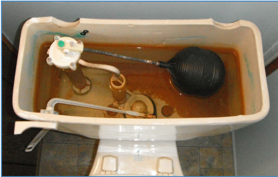
Photo 1. Iron stains in toilet tank.
