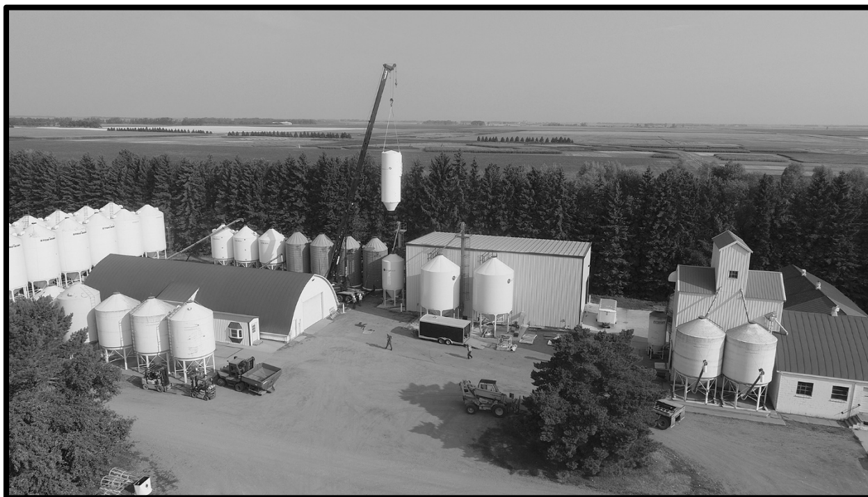
UAS-view of the crane moving the seed mill dust system into place.
