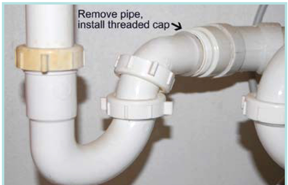
Figure 16. P trap under sink.
