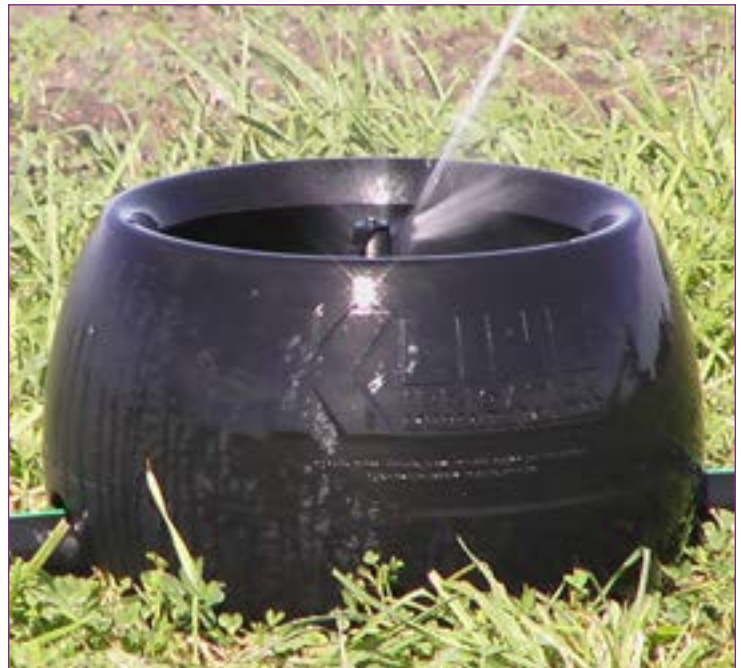
Figure 3. A moveable sprinkler irrigation system applying containment pond effluent
