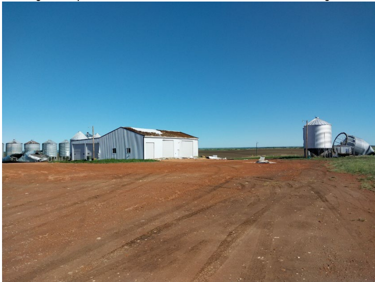
Figure 2. Damaged silos in Mercer County. Photo: Craig Askim, NDSU ANR Extension Agent.
