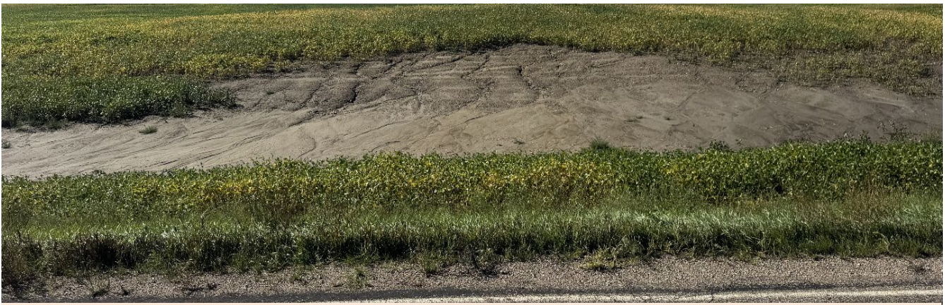
Figure 5: Severe water soil erosion from heavy rains in Griggs County on 9-4-26.
