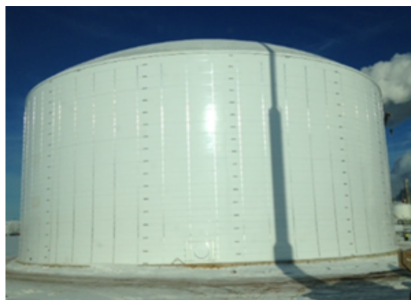
Figure 28.3 An 11-million-gallon capacity refrigerated and insulated ammonia storage tank at Dakota Gasification facility near Beulah, ND.
