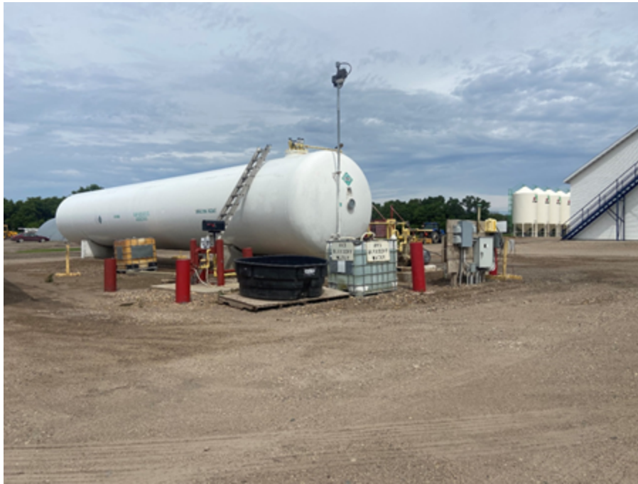
Figure 28.2 Ammonia storage at retail fertilizer dealer location, Arthur Companies, Arthur, ND. Note the black tanks used for emergency water storage the concrete barriers that prevent plumbing accidents from vehicles, the multiple pressure relief valves on storage tank top, and all of the proper signage prominently displayed on the tank. The platform for loading nurse tanks is on the opposite side. Image used with permission.
