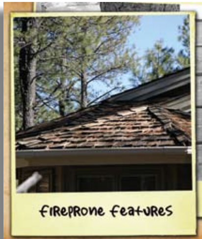
Use of flammable roofing materials
