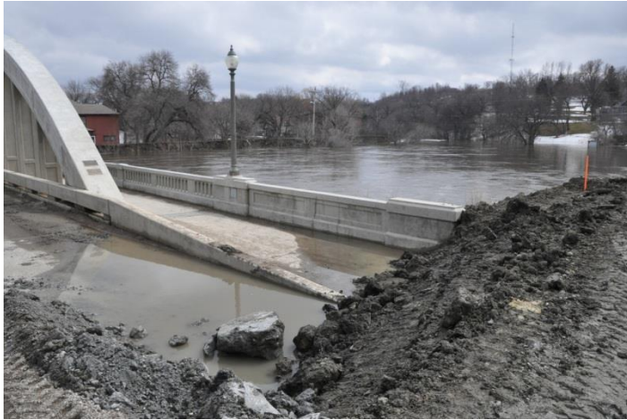
Photograph 10.4 Valley City Rainbow Bridge during 2009 Flood Source: Public Domain , www.fema.gov/photodata/original/40696.jpg
