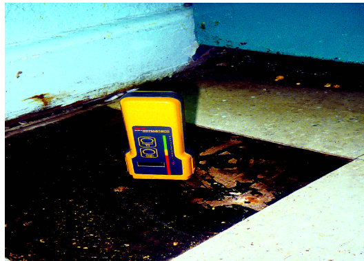
Photo 2: Extensive mold contamination of ceiling and walls
