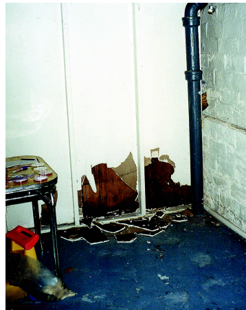
Photo 3B: Front side of wall-board looks fine, but the back side is covered with mold
