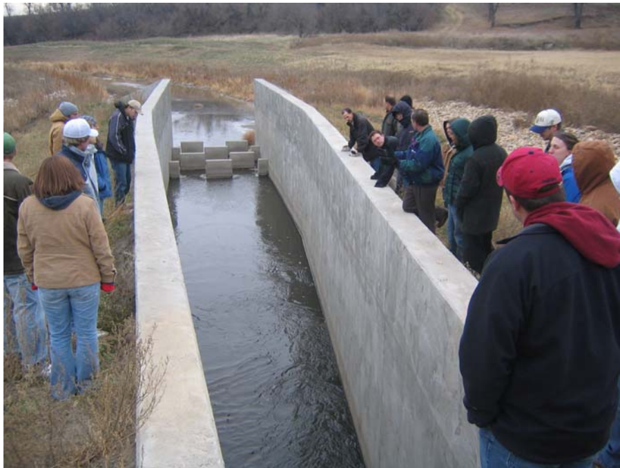
Pipe outlet structure of Maple River dam under low flow conditions. Some of the WRRRI Fellows along with hydrology course students from NDSU are taking a tour.
